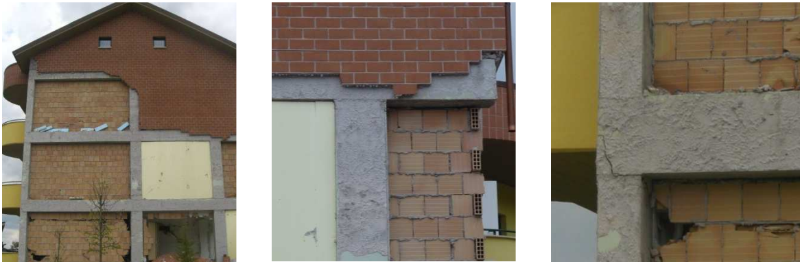
Figure 2: Total disconnection of the outer veneer cladding wall.
