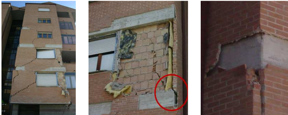
Figure 1: Cracking and collapse of the outer leaf of a double leaf wall.
