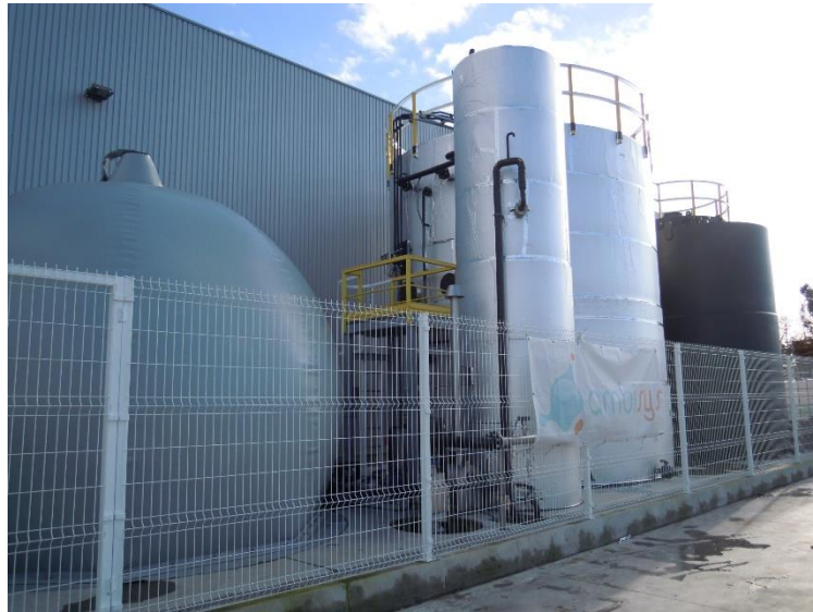
Figure 7: Poveira industrial wastewater treatment plant (Ambysis).
