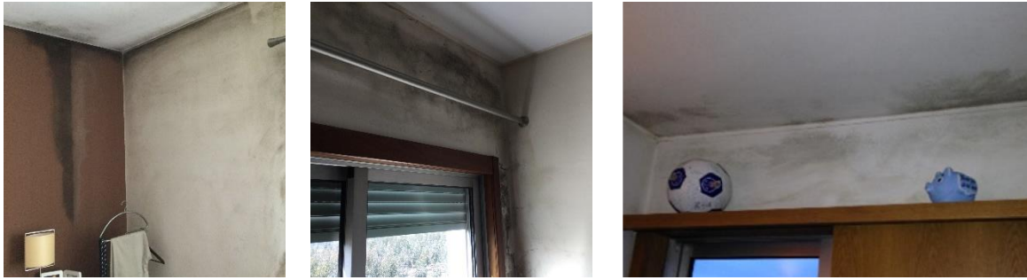
Figure 2. Examples of observed anomalies (condensation, humidity).
