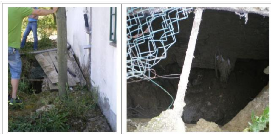
Figure 2. Location and view of the detected instability - land clearing up to about 5.0 m (Henrique, 2017).
