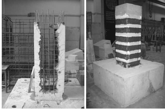
Fig. 12 Hollow square section pier (PO1) before and after the shear retrofitting with CFRP sheet
