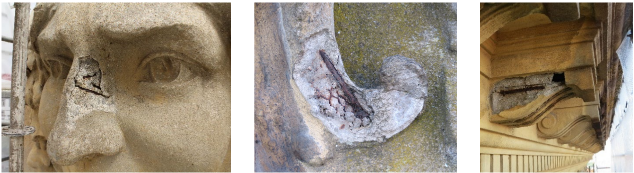
Fig. 7. Examples of damaged reinforced concrete decorative elements of the façades of the São João National Theatre.
