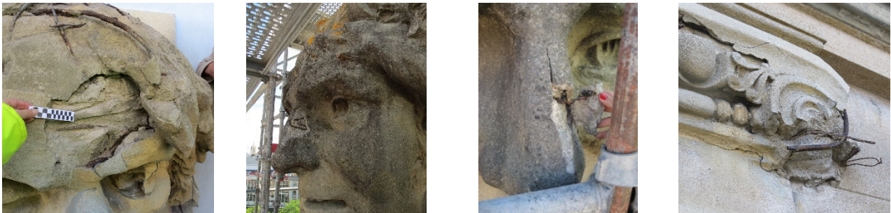
Fig. 1. Architectural sculptures in reinforced concrete with material degradation resulting from corrosion of the reinforcement.
